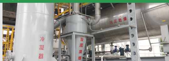
Sludge Drying System
