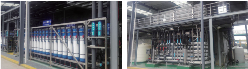
Facility for recycling reclaimed water at Far Eastern Dyeing & Finishing (Suzhou) Ltd.
